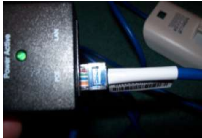
Figure 12 – Cabled from device connects to "POE"
